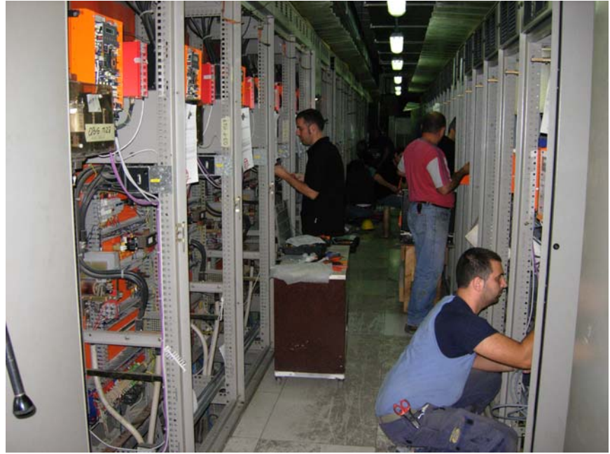
Electrical wirings made on site by SAEL
