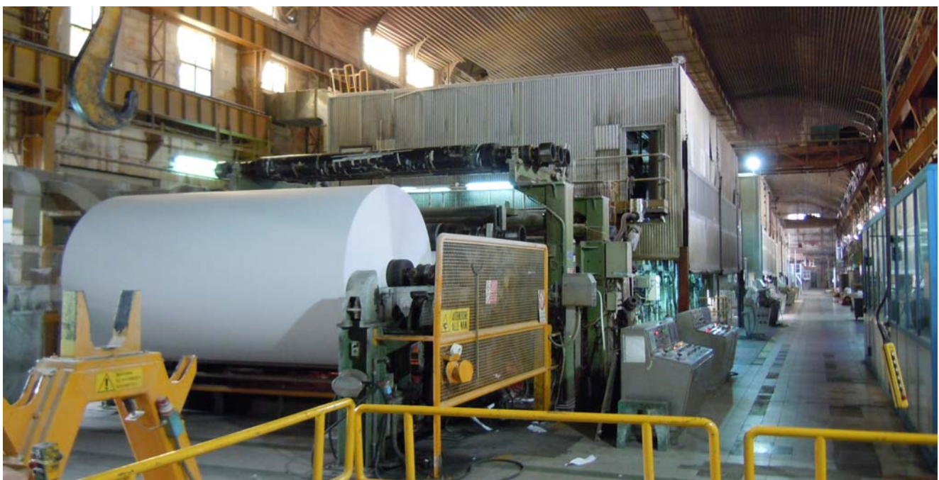
AVEZZANO PAPER MILL, FINAL SECTION CONTINUOUS MACHINE, SAEL Intelligent Drive
