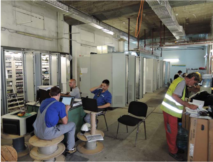
MEL papermill, Drive and automation room during commissioning
