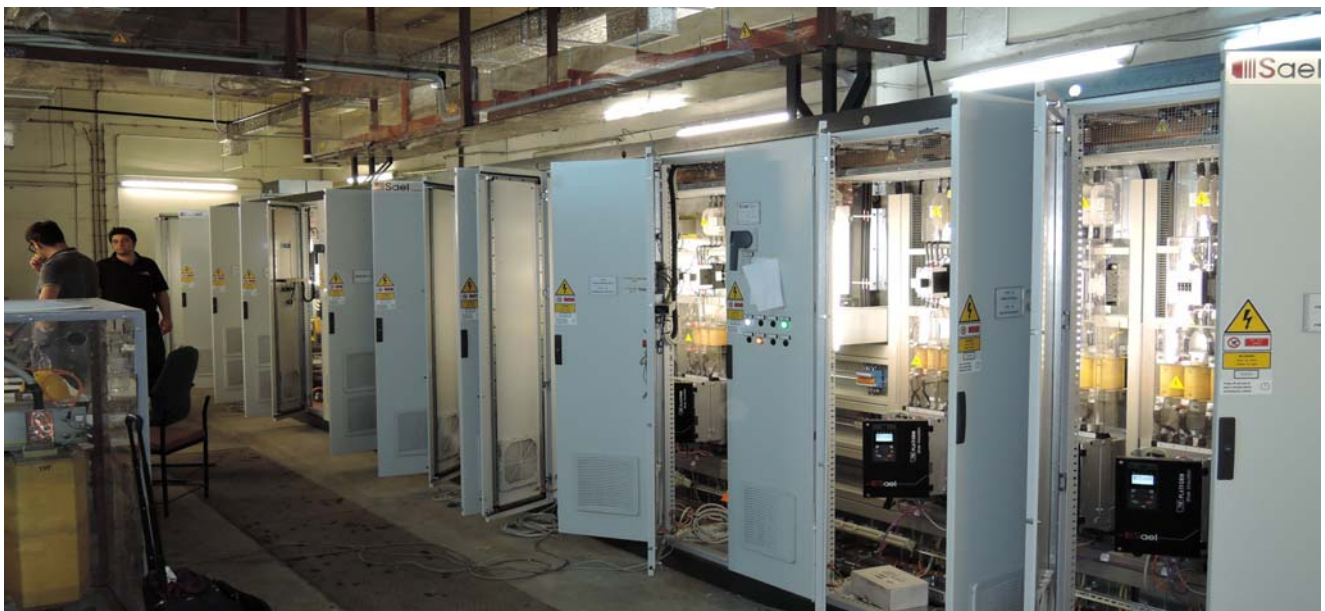
MEL cabinet room, combined with double side mounted drive to reduce the space.
