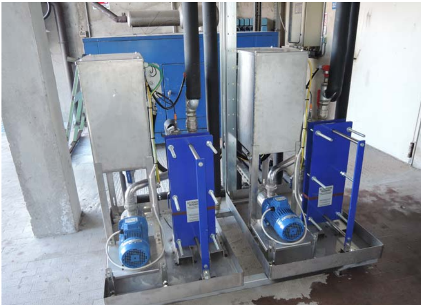
Water-water heat exchanger - direct supply from the well of papermill for cooling inverters and electrical panels
