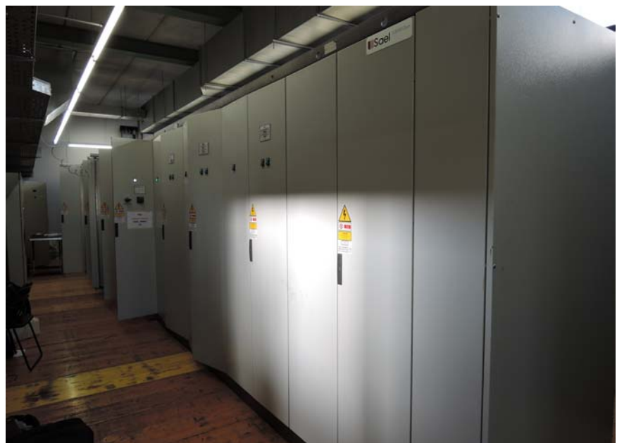
Electrical cabinet dry section with inverters cabled in double side and with water cooling.
