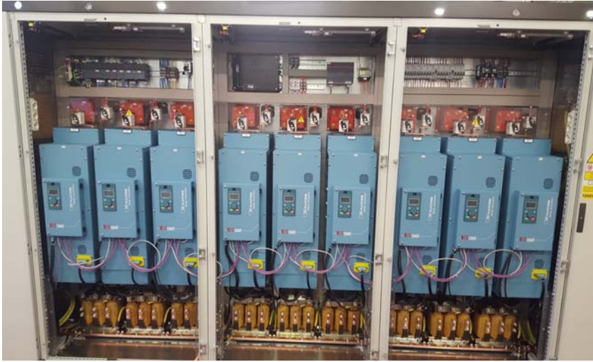
9 inverters of 400KW cooled with water in cabinet of 3 mt, cabinet of Tunnel Boring Machine - ONE DRIVE WATER.
