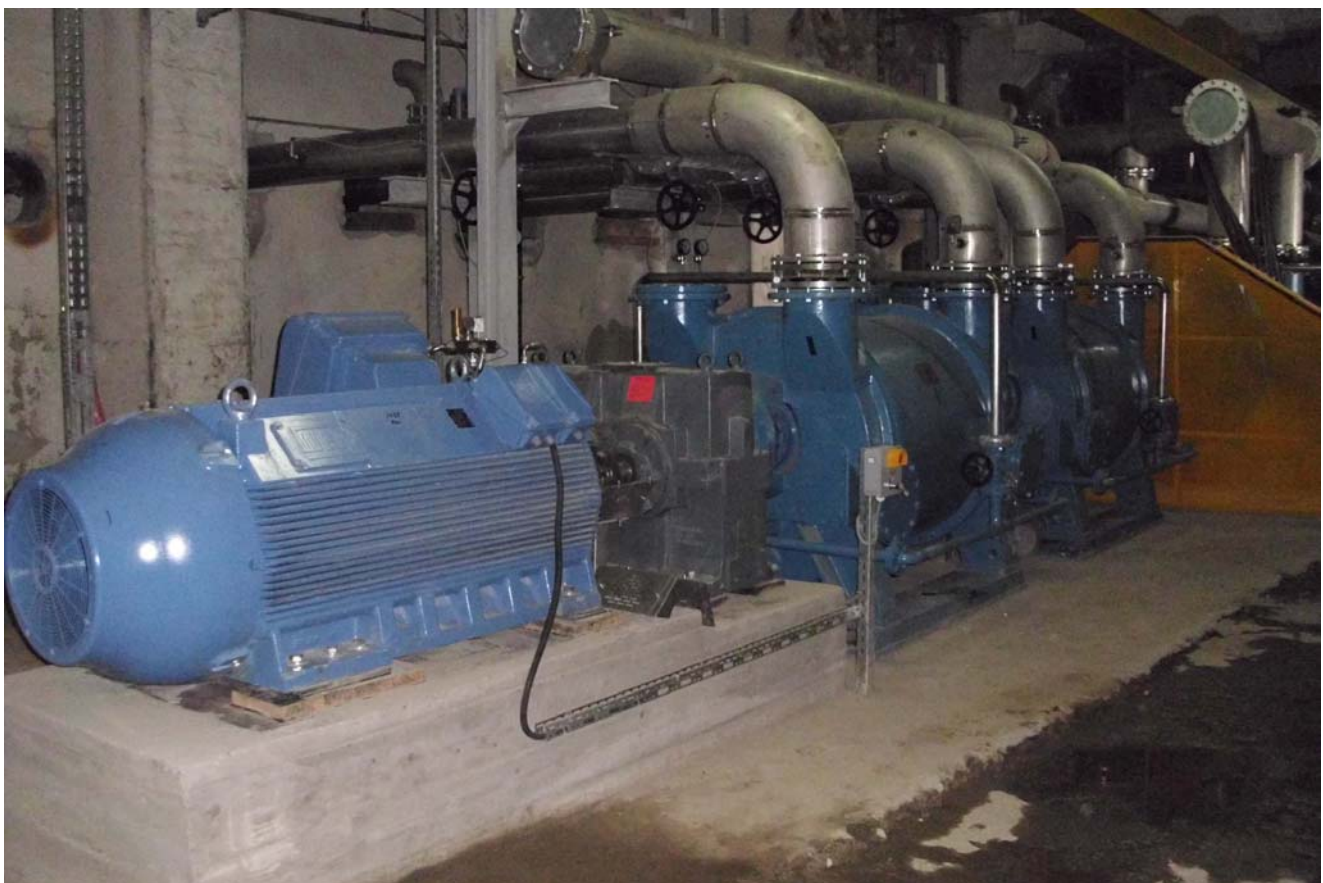
Typical Cutes Europe installation with series of pumps for felts conditioning
