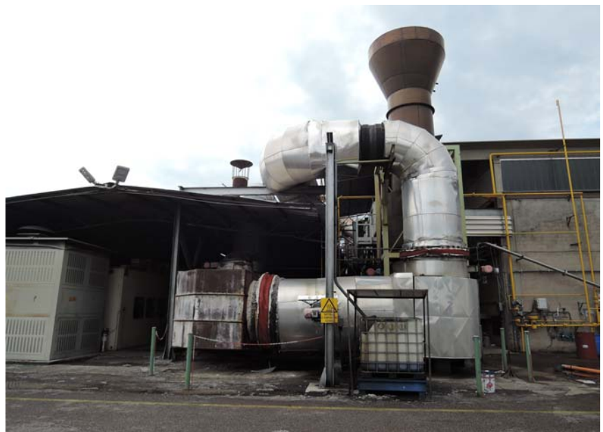
Global photo of Turbogas 5Mw reconstructed at Cartiera Vignaletto.
