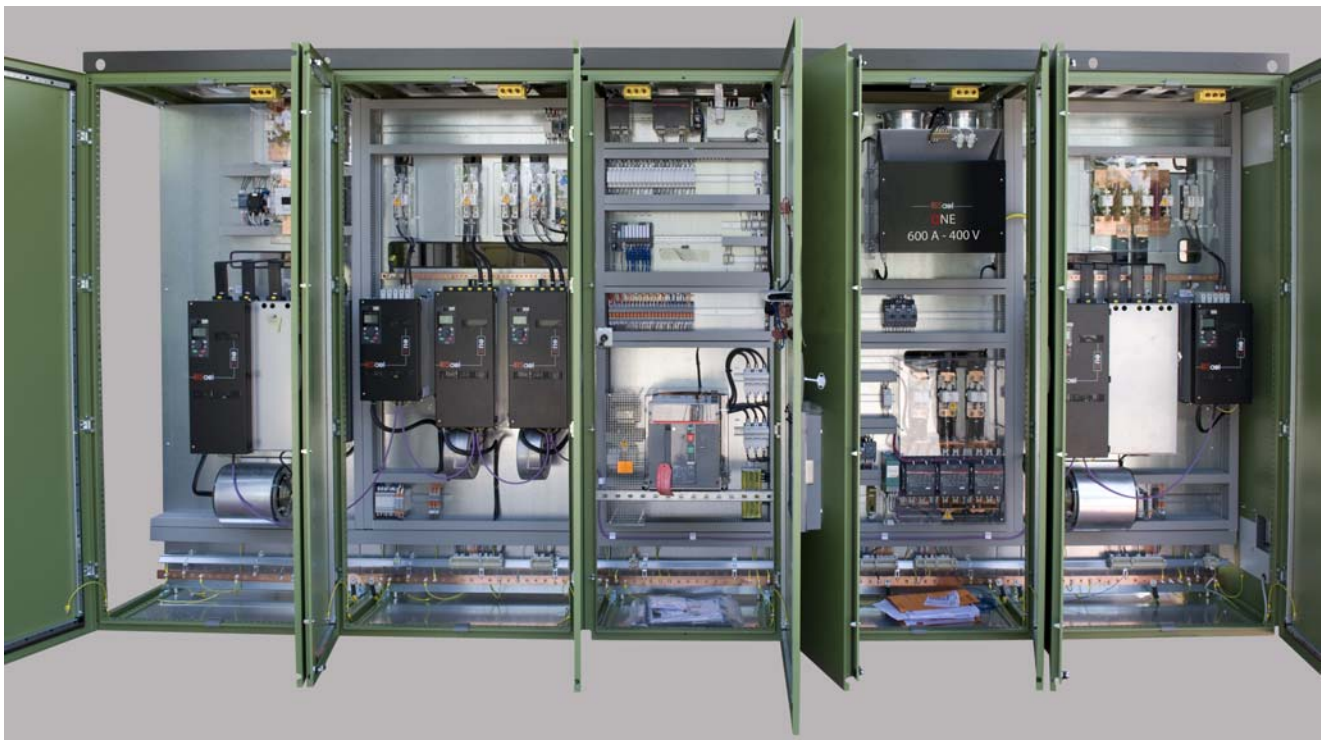
Sectional drive with “PLATFORM ONE DRIVE” Inverter Electrical Cabinet.
