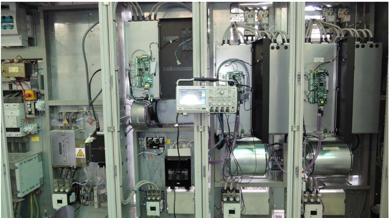
Syncro Jagemberg Electrical Cabinet – Next Gen after the rebuilding – Sarego, Burgo Group
