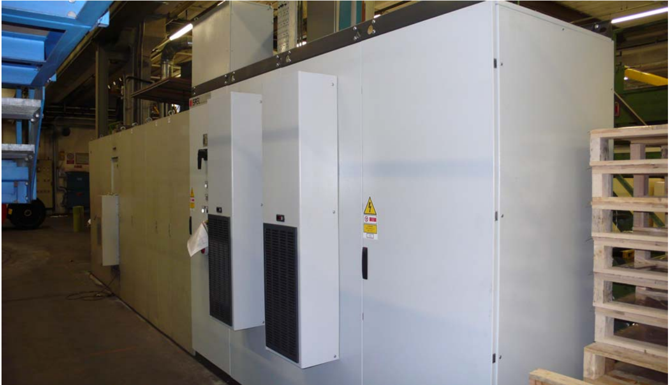
Sheeter electrical equipment after the taking place of the new AC equipment vs. the old Jagemberg cabinet
