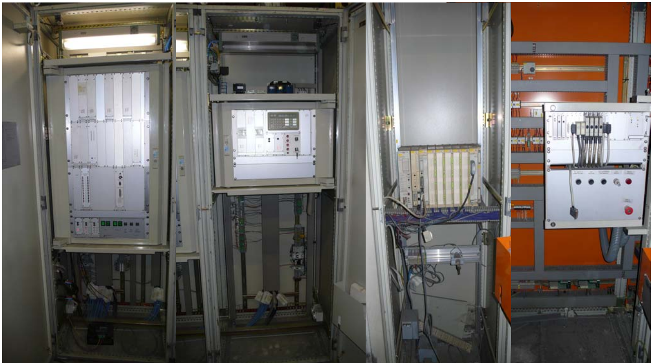
Jagemberg DQA electrical cabinet sections and knife control before the revamping: All the electronic board were replaced as much as the S5 PLC with a S7 PLC. The Micromatik motor drives and knives were replaced by a new electrical equipment with AC inverter - substitution of the old DC management driven by a Micromatik micro processor.
