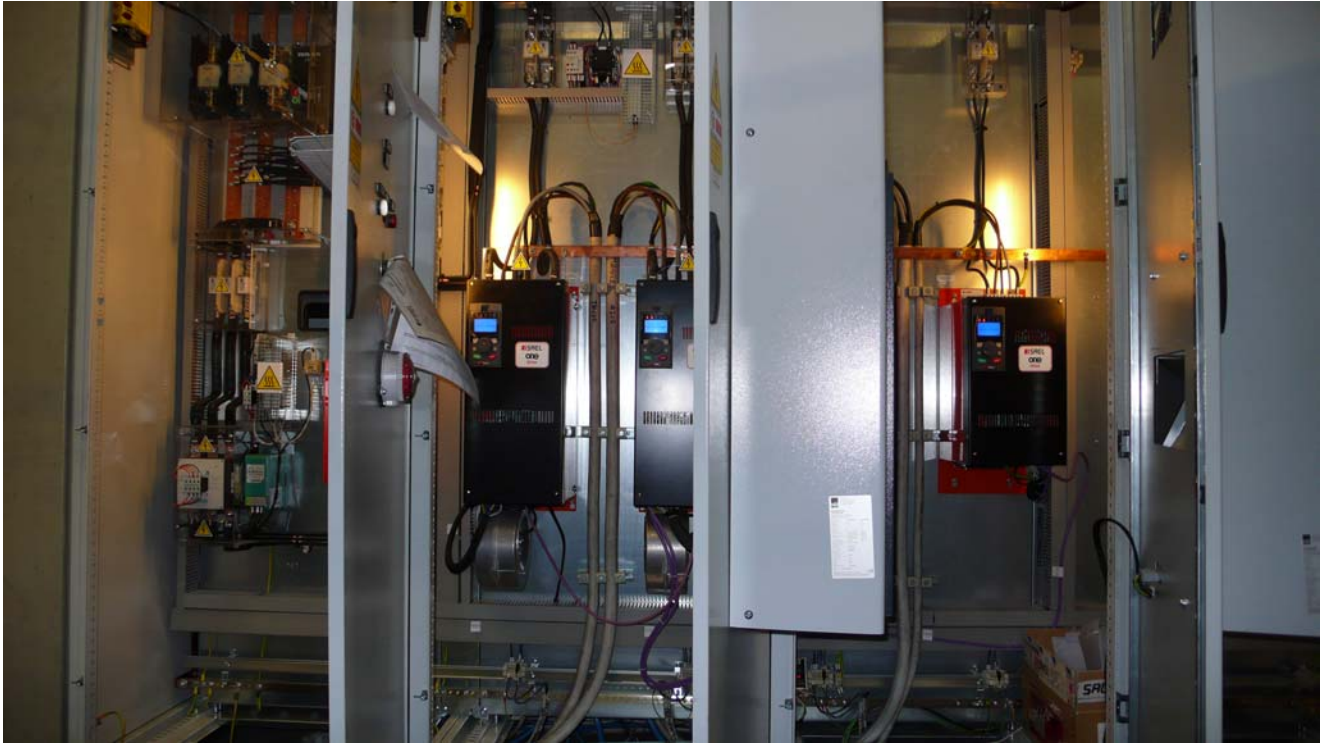
View of the new electrical equipments with ONE Inverters who replaced the old DC drives ; the knife electronic management is made by the ONE board within the SAEL drive. Out of the "PLATFORM ONE" drives no other hardware or electronic boards were used.
