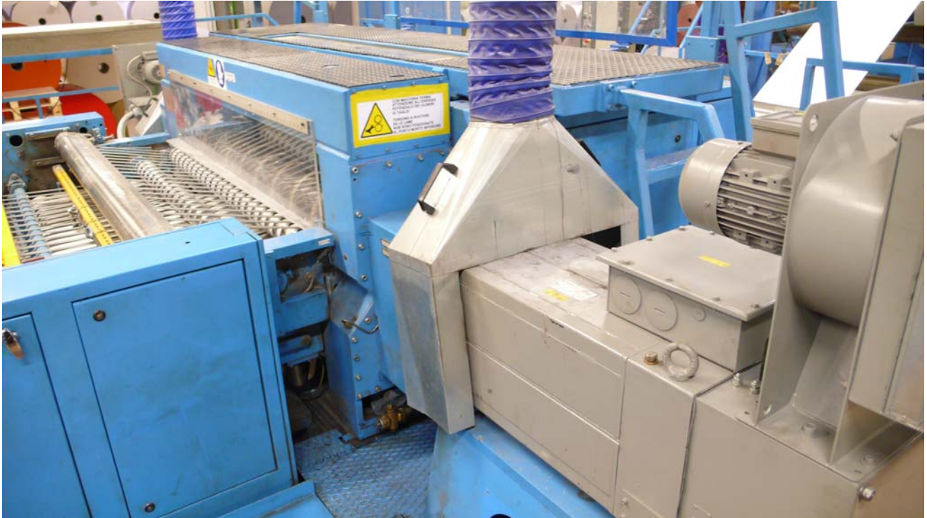
The STOP AIR motor management and the knife - in DC before - have been replaced by equivalent AC motors driven by ONE DRIVE inverters. The Favini's team made the mechanical replacement by them selves.
