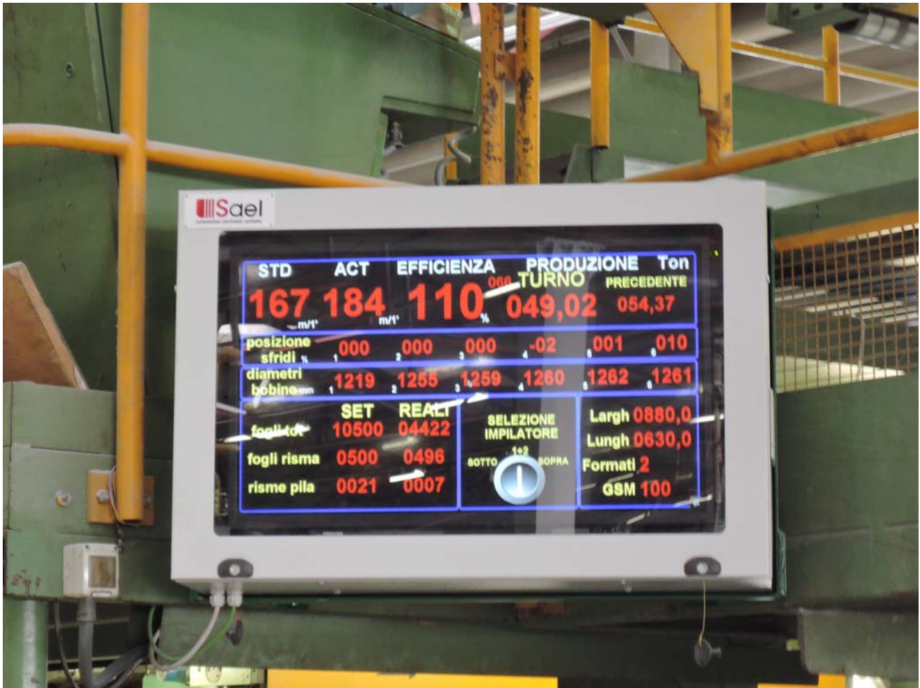
The new monitor 40" to show the production data of the sheeter, Cartiera del Garda.
