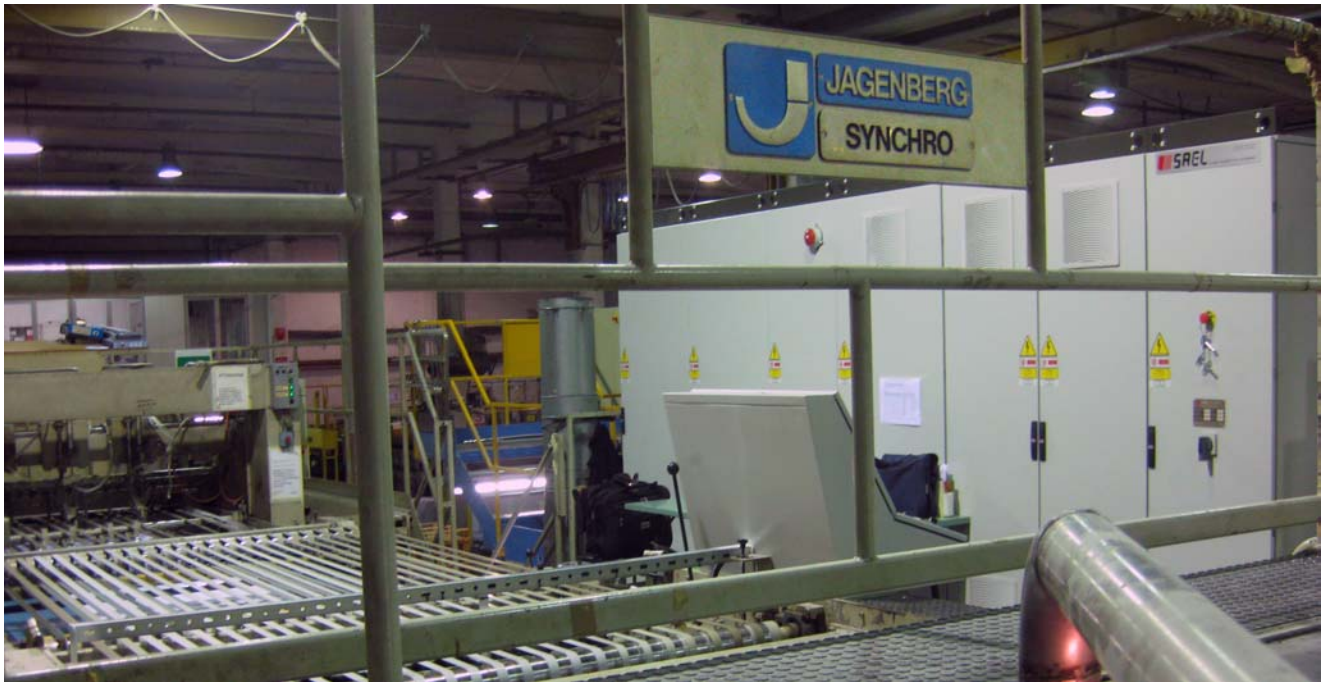
View of cutting area – Jagenberg Synchro sheeter rebuilt with new cabinet, drive and automation
