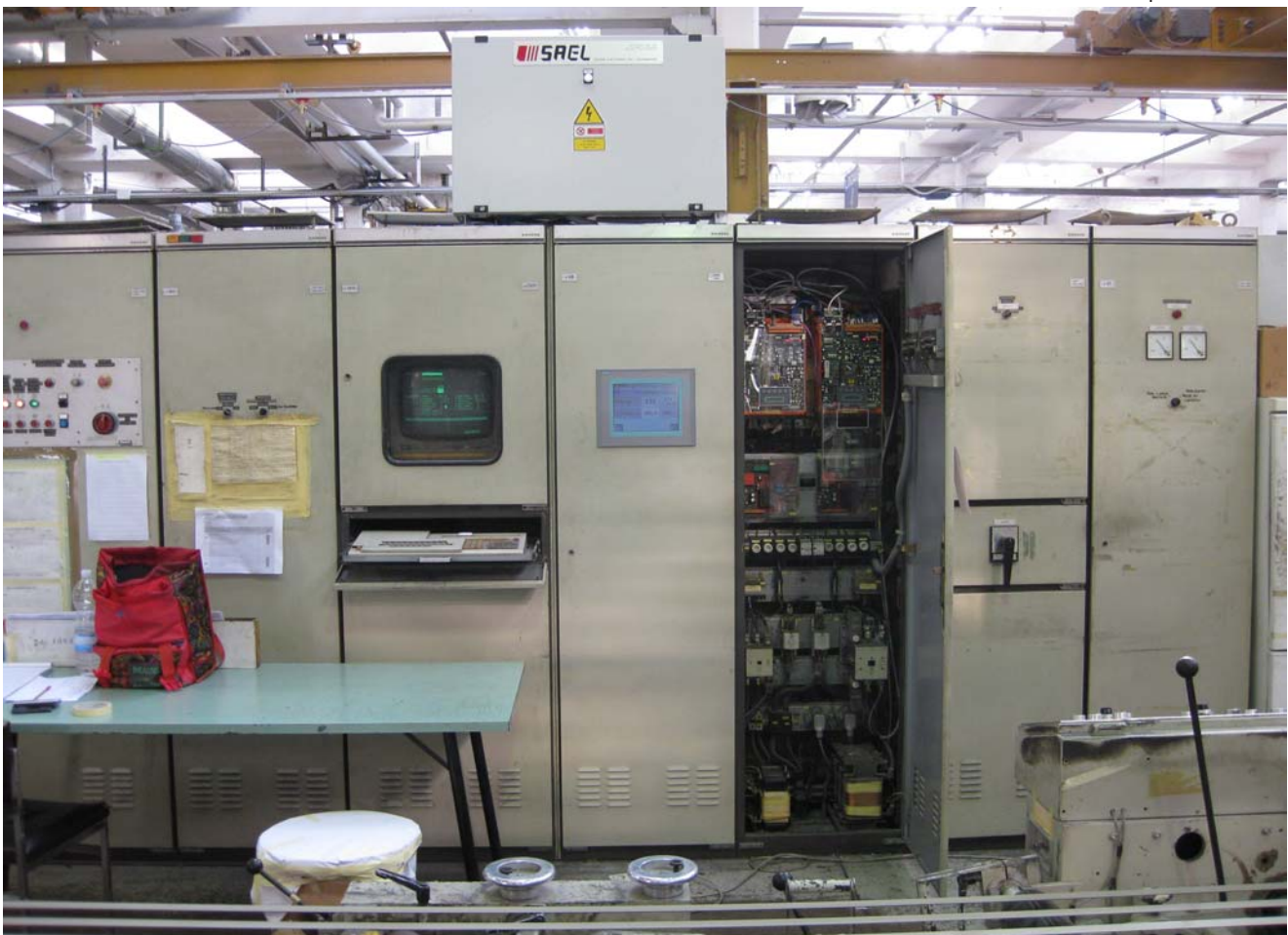
View of the complete cabinet after the emergency restart -Step1-
