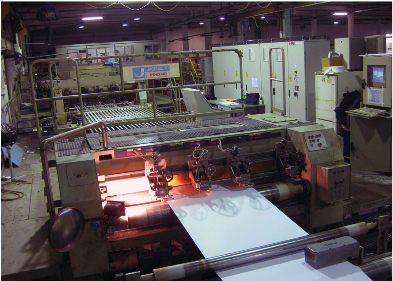
View of rebuilt Jagenberg sheeter with new electrical cabinet - Burgo Toscolano papermill
