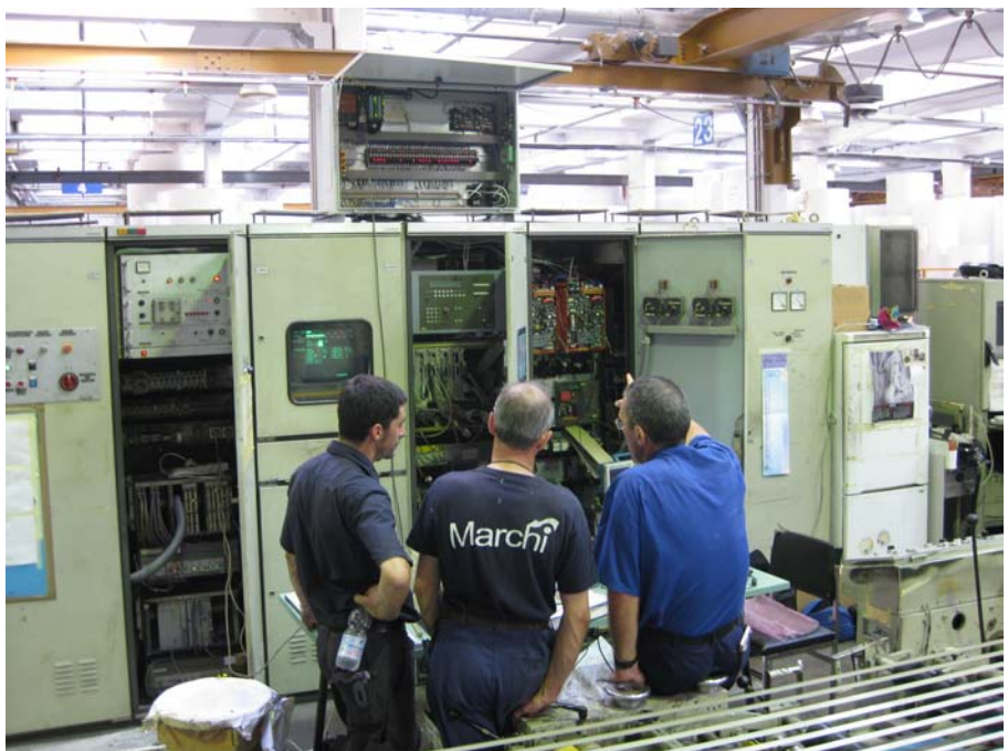
Electrical cabinet of Jagenberg Synchro, Burgo Toscolano step1 emergency
