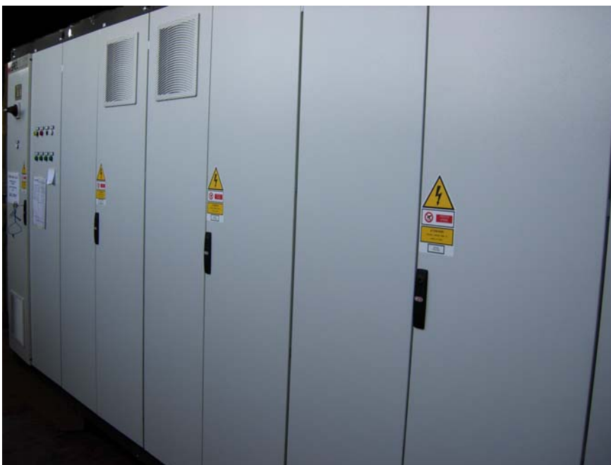
New equipment - Replacement of the old electro mechanic part
