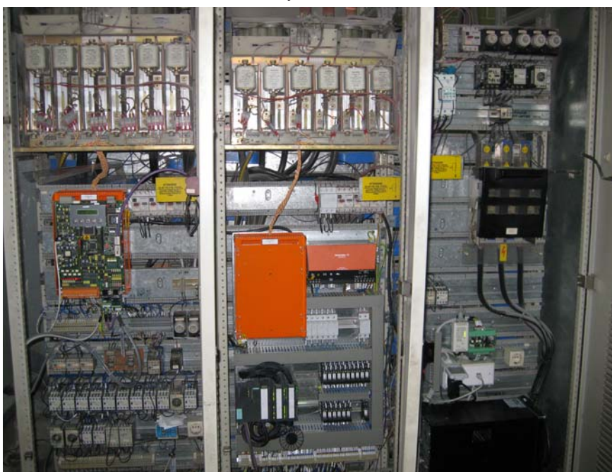
Unwinder Siemens Drive restarted after the modification
