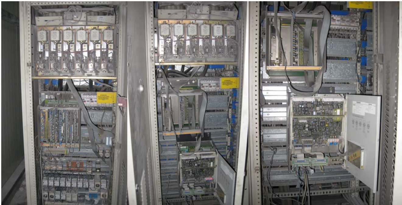
Old Siemens Drive before the modification and the “Reborn” replacement
