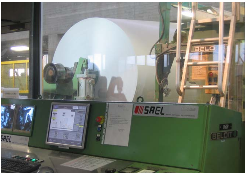
Drive Control Desk before and after the electrical modificaiton
