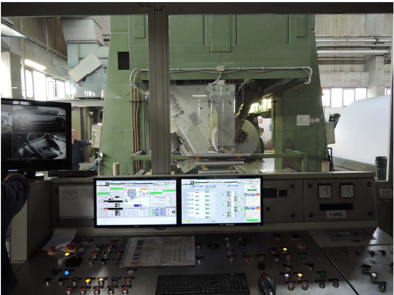
Winder Main Drive with DCS “WINDER SAEL” – Redundancy and Touch version upon demand
