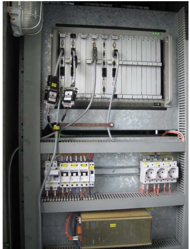
TECNINT Rack and dismantled regulation boards
