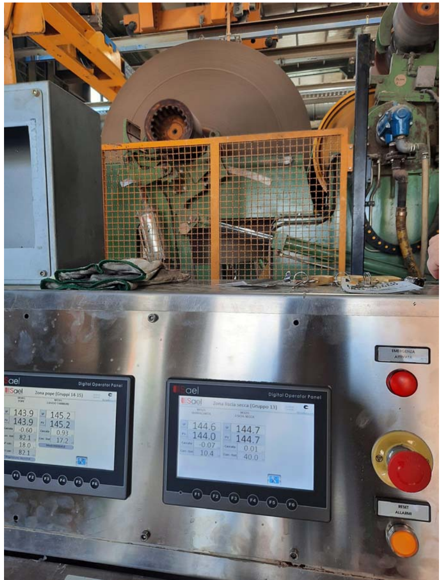
Pope Control Panel
