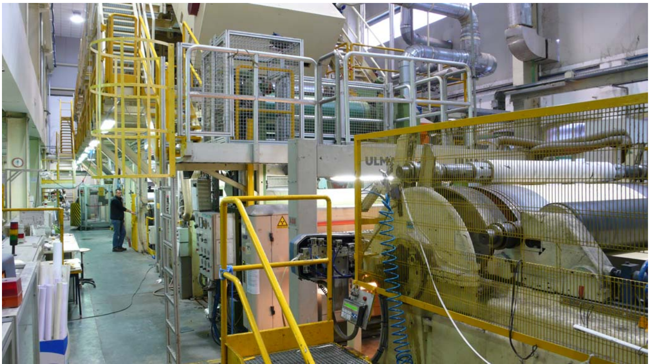
CORDENONS PAPER MILL, coating machine 2 in line with sinchro electronic cutting machine
