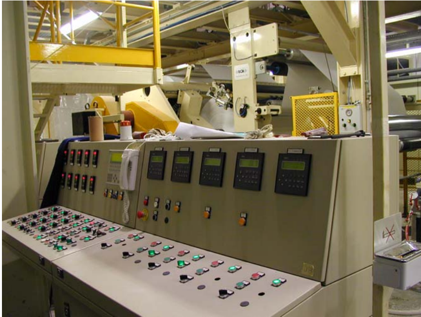
COATING 2 UNWINDERS CONTROL BOARD, CORDENONS GROUP.
