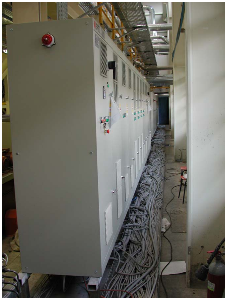
COATING 2 CONTROL EQUIPMENT, CORDENONS GROUP.
