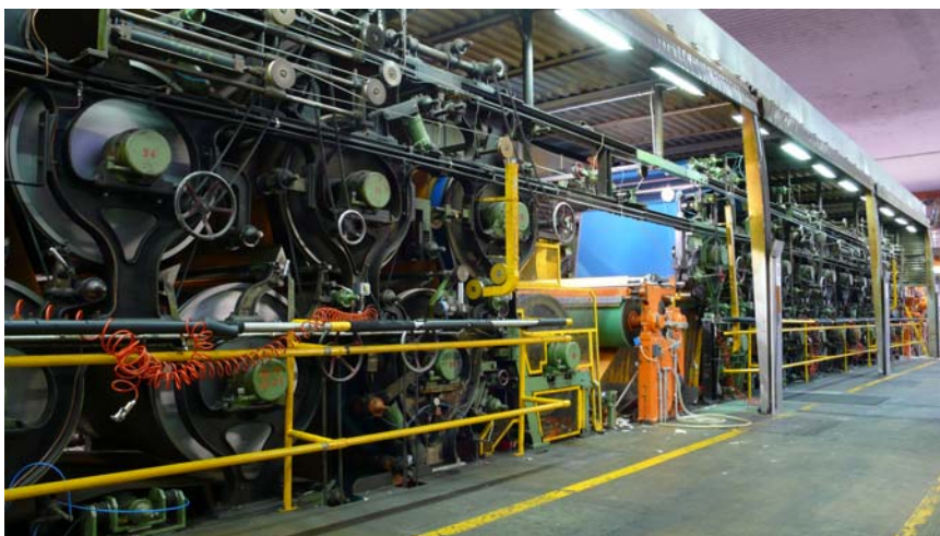
View of PM1 pope zone and size-dryers, wer the single-shaft was eliminated substituting it with new AC sectional drives
