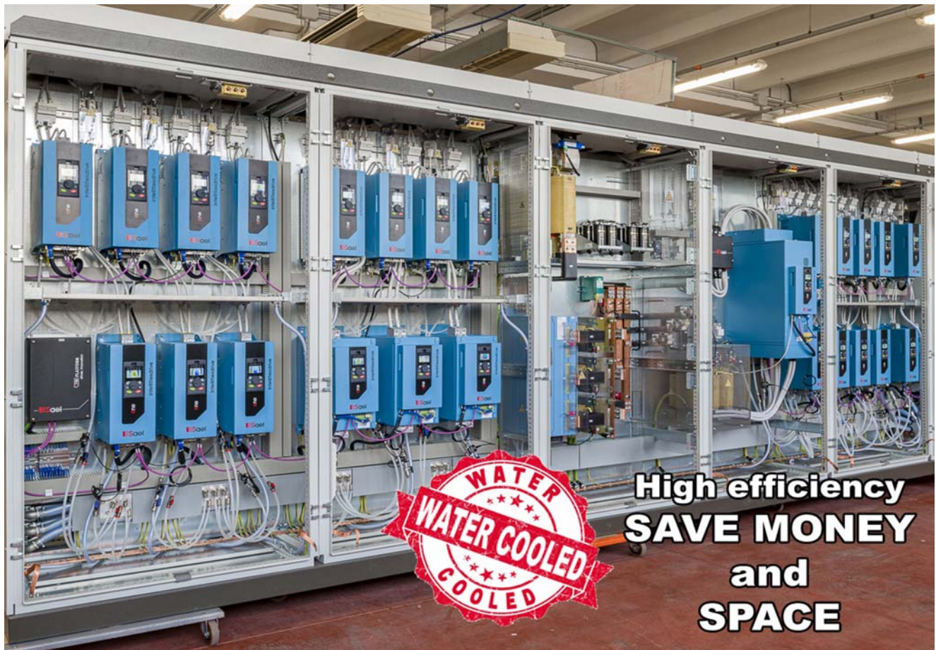
Electrical cabinet with inverters cabled in double side and with water cooling.
