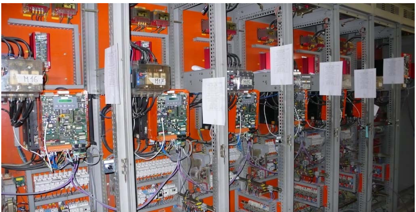
Old electrical cabinets revamped by the “REEBORN” – Archive images -
