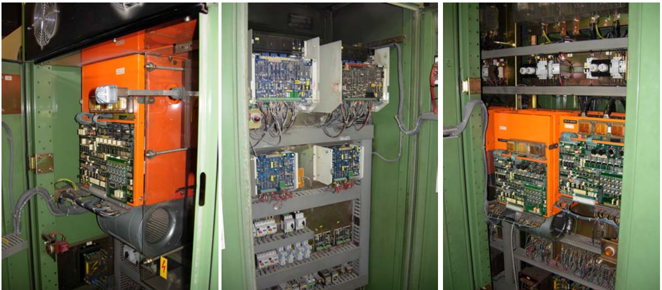
Existing cabinets view before the “REEBORN” revumping
