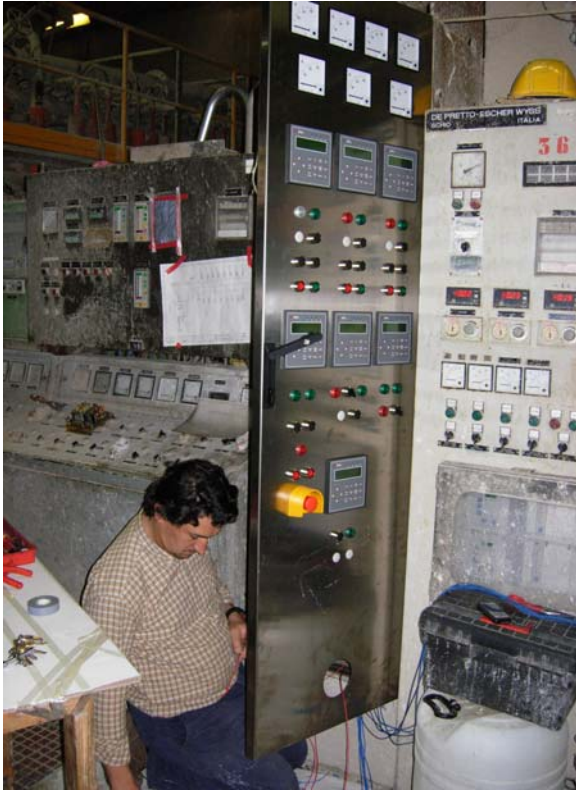
Cabling inside Papermill of the new cabinet-desk to control the wet area
