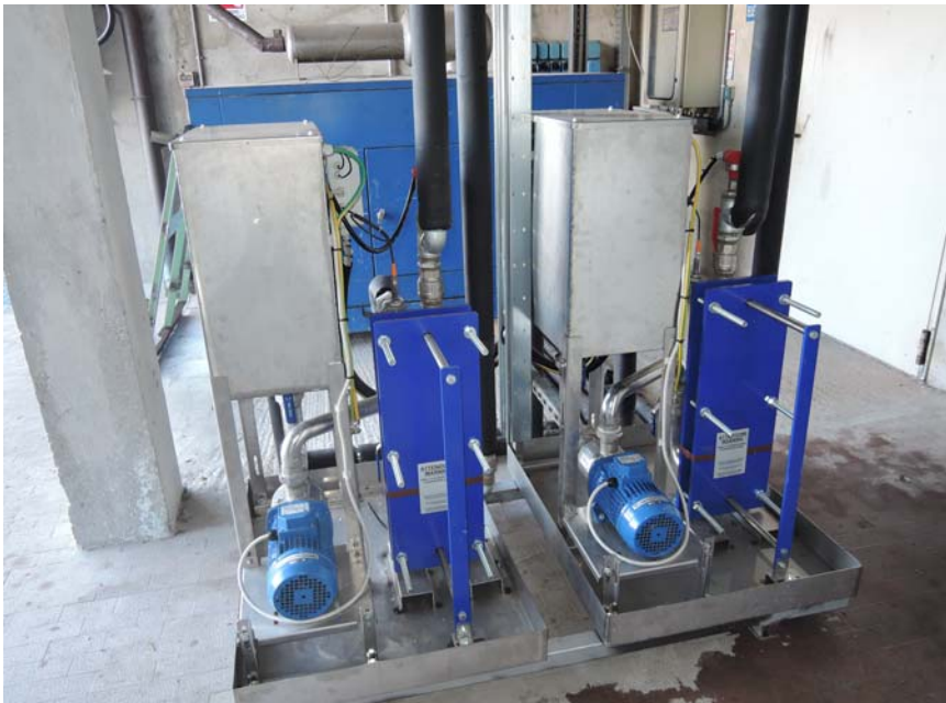
Water-water exchangers with direct in-let from the well of water
