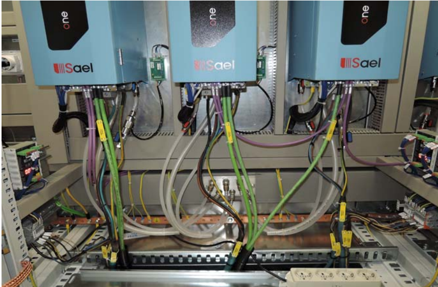
Sectional drive electrical cabinet by the exclusive "PLATFORM ONE" drives WATER
