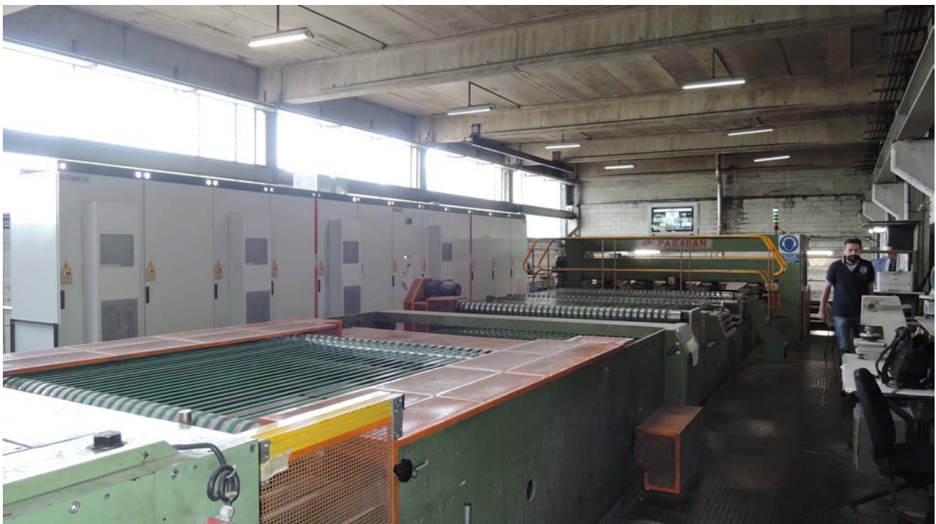
Electrical cabinets, automation, and sheeter control after the modification; electrical cabinets renewing with mirroring mounting execution (providing all the electrical connection as it was).
