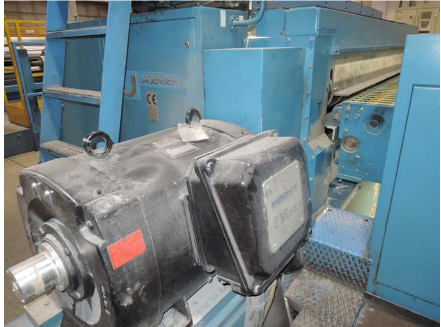
The existing Micromatik AC motors are driven by the SAEL ONE Drive Inverters
