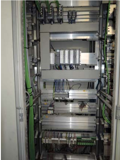
S7 300 Siemens PLC re-wired vs. the former S5 115 model
