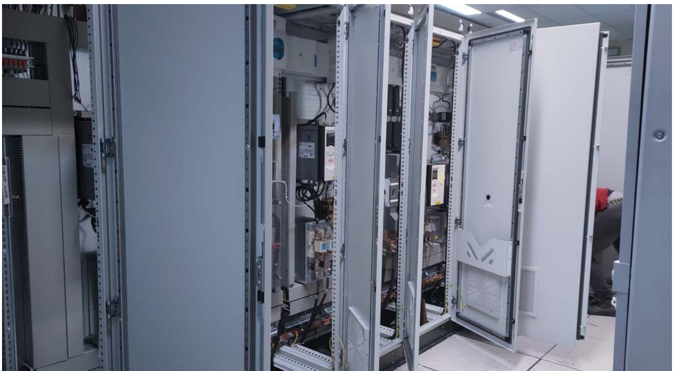
Electrical cabinet of Automation and Drive using ABB DC DRIVES.
