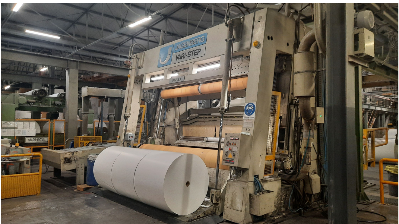
Jagenberg VARISTEP rebuilding: after 7 days of start-up, the first lifting, immediately judged satisfactory - PLATFORM ONE DRIVE SAEL
